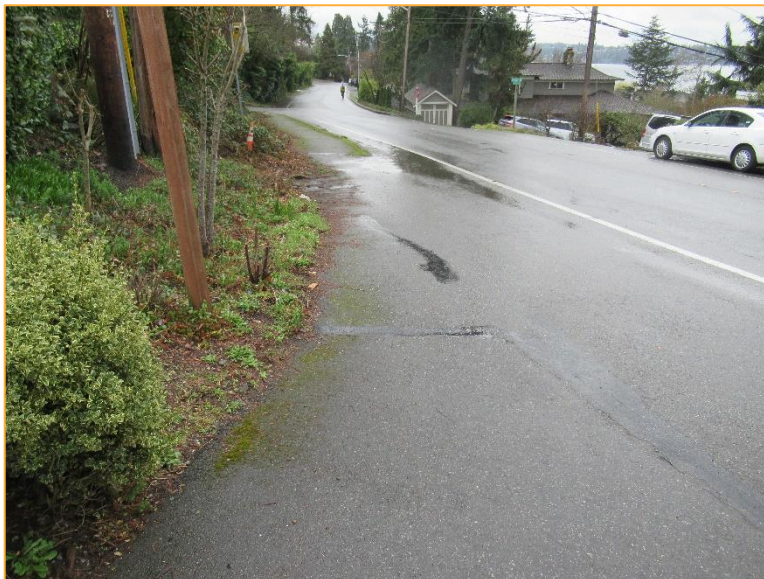
Photo 6 – Facing south at the general location of catch basin 18c-24 which could not be located during field investigations, presumably because it was completely covered by debris and vegetation.
