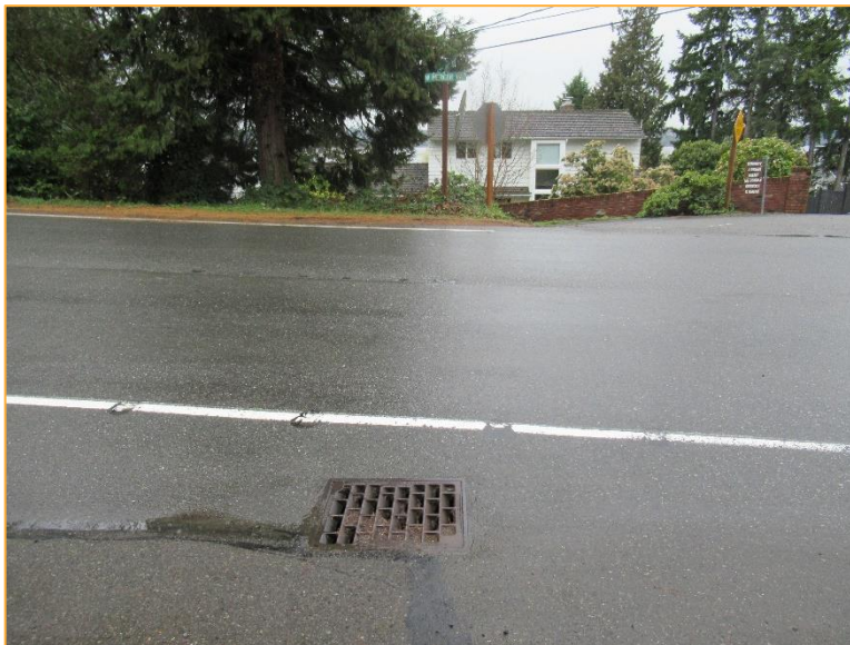
Photo 10 – Facing southwest at catch basin 18c-143 which redirects the stormwater across West Mercer Way and down the branching 67 th Ave SE.
