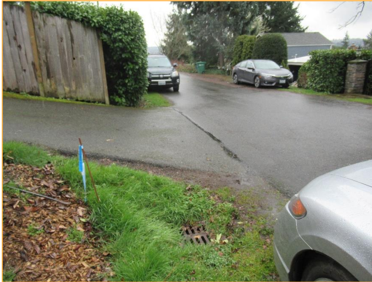
Photo 3 – Facing southwest, the next catch basin (18c-27) immediately downstream from the entry point. Stormwater continues to flow southwest along 67 th Ave SE.
