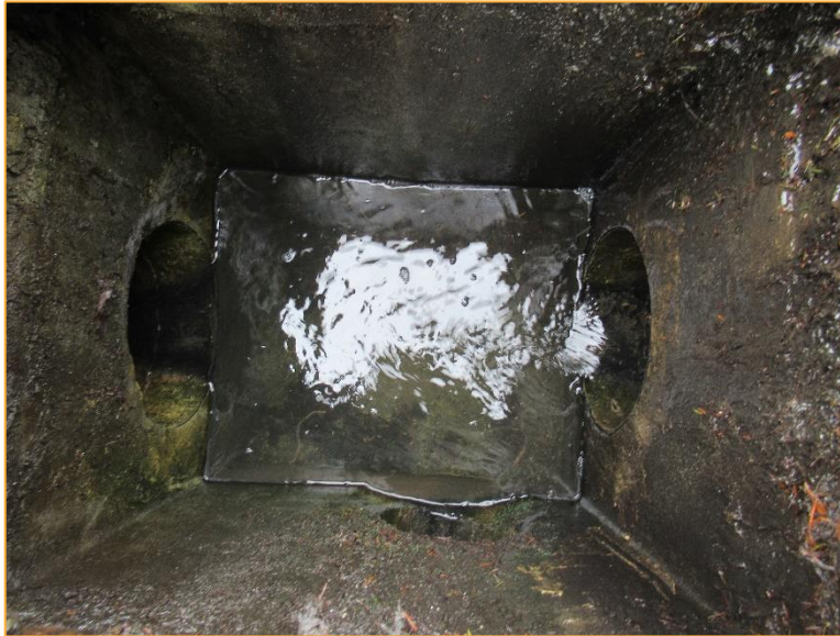
Photo 7 – Inside of catch basin 18c-6, directly downstream from catch basin 18c-24. Flow volume consistent with adjacent catch basins indicate limited to no blockade from debris covering catch basin 18c-24.
