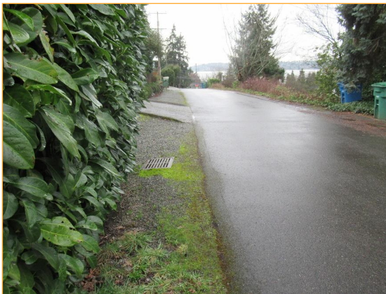
Photo 4 – Facing southwest, this is catch basin 18c-21, immediately downstream from catch basin 18c-27. Stormwater continues onto catch basin 18c-22 and then to 18c-23.
