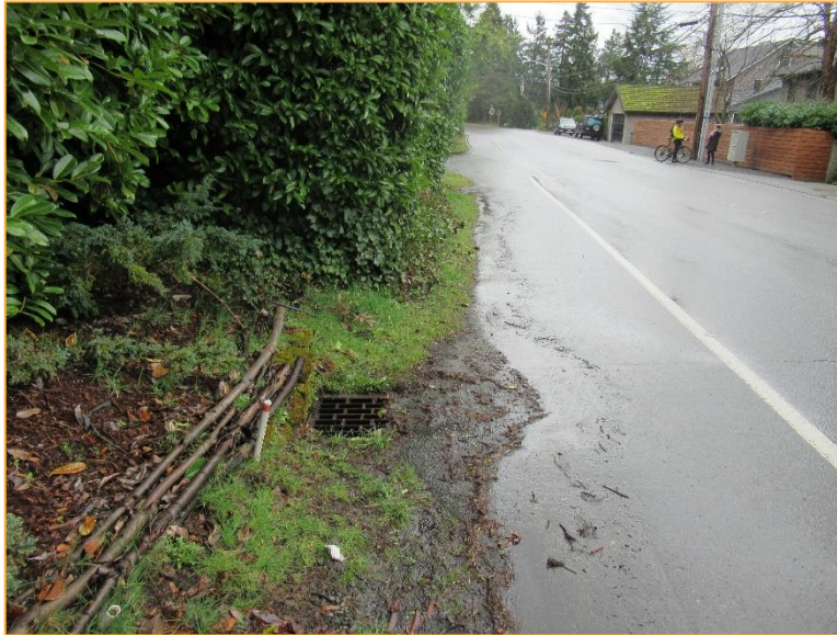
Photo 9 – Facing south at catch basin 18c-140, directly downstream from catch basin 18c-11. Stormwater continues south through catch basins 18c-16, 15, 17, 141, and 143 in that order.
