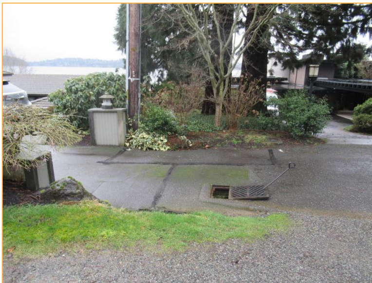
Photo 12 – Facing southwest at catch basin 18c-163 which redirects the stormwater across 67 th Ave SE and down an easement along the southern property line of parcel #3708900070 until discharging directly into Lake Washington. Strong flows indicate no blockage.
